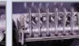
Emergency control valve can be controlled from above and flow stopped in case of emergency
